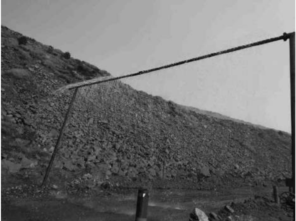
Over Head Dust Suppression Arrangement installed at Haul Road for wetting the coal loaded over trucks
